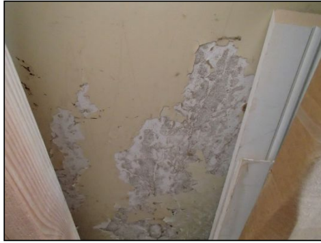
termites ate the paper off of the drywall
