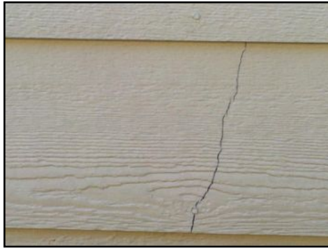
Siding was damaged.
