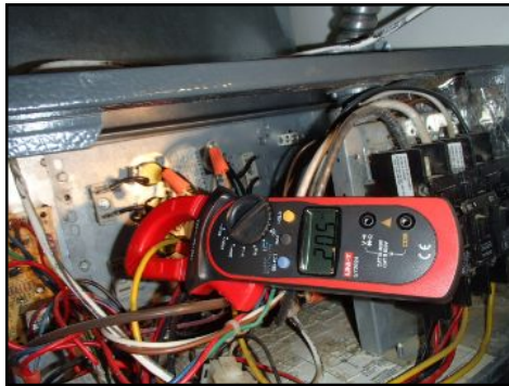
Backup electric heat was operable.
