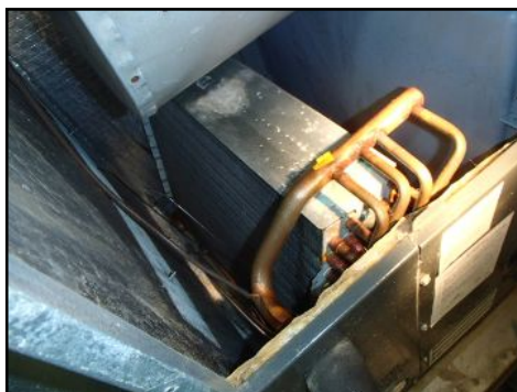
Evaporator coil was operable.
